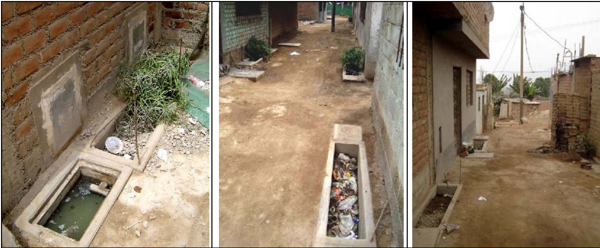
Figure 5: Deficient and no maintained sand filter in Nievería
