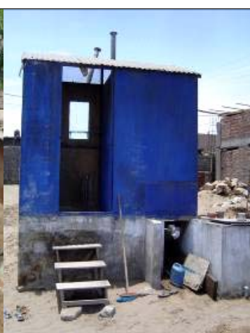
Figure 3: Two chambers dehydration and urine separating toilet
